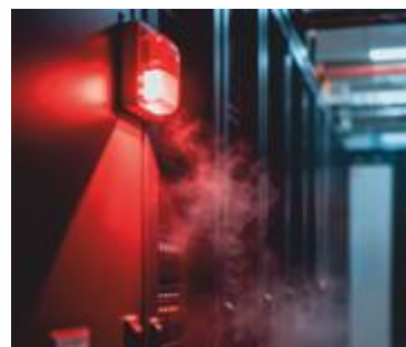
Fire Alarm System
